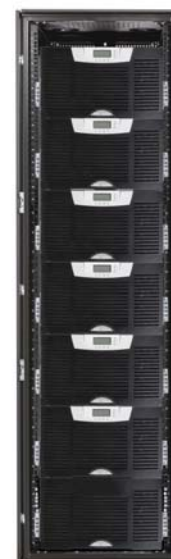
Powerware BladeUPS in a rack (60 kW, N+1 Redundant)
